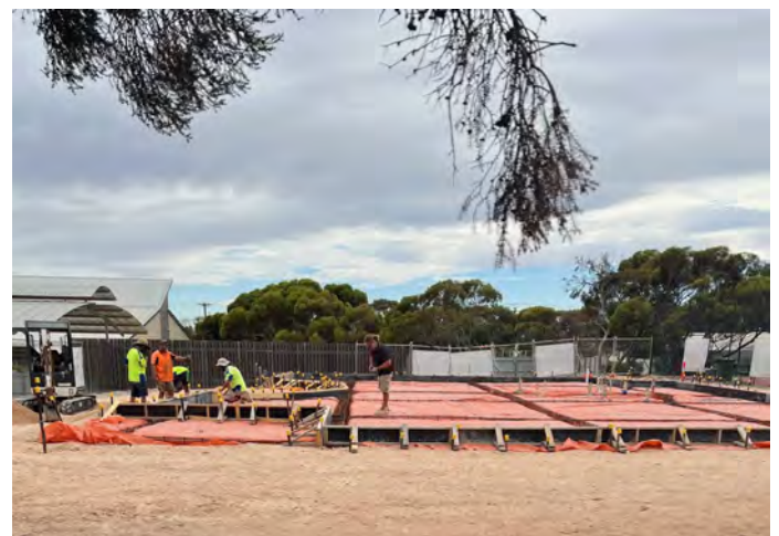
Above : Exciting times. Building of our Wellbeing Hub is progressing – Concrete being poured next Monday.
